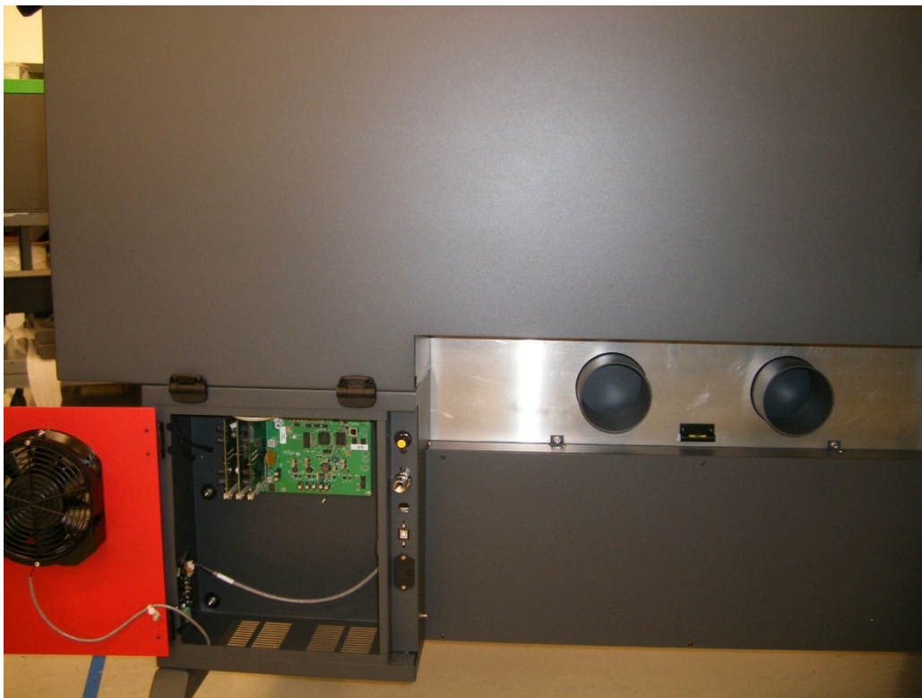
CPU Cabinet where automation kit is to be installed
